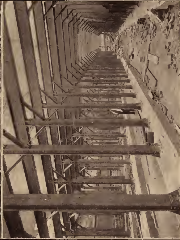
TUNNELING LOWER BROADWAY. Temporary roof for surface traffic in daytime. STEEL STRUCTURE of four-track sections, 50 feet wide, 13 feet high. Water-tight linings.
